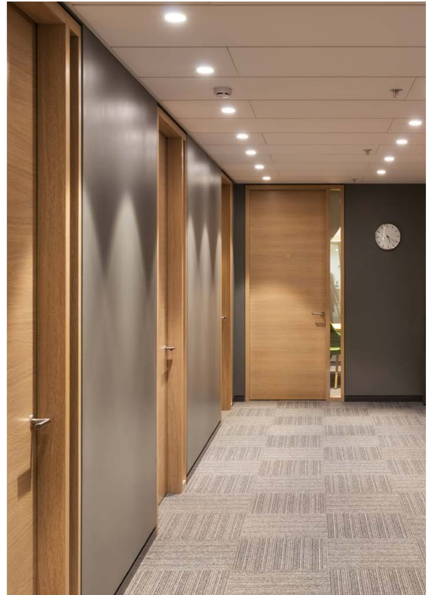
Application of RQ 160 LED in corridor.
